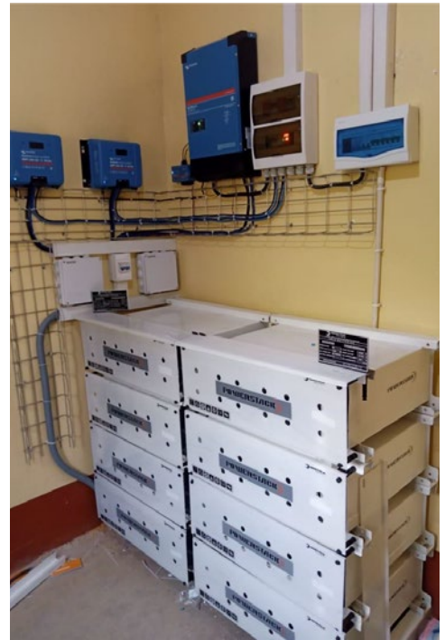
Picture 1: Inverter, charge controller and LI-batteries
