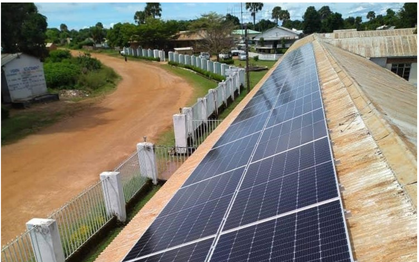
Picture 2: Photovoltaic modules on a hospital roof
